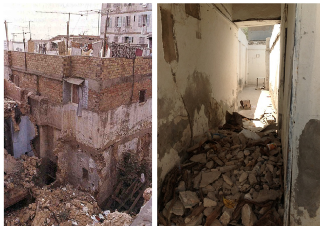
Fig. 1 Advanced state of deterioration in the Casbah of Algiers, Algeria, and Al Asmakh historic district in Doha, Qatar in search of immediate rescue.
